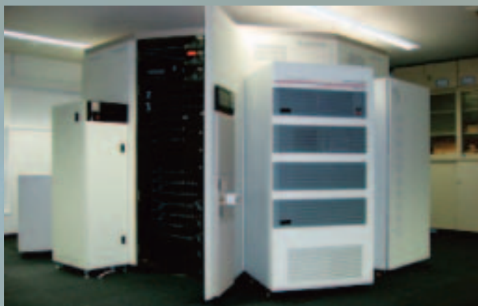
Figure 1. 500Tera-byte data archive system at the Institute Industrial Sciences, University of Tokyo
