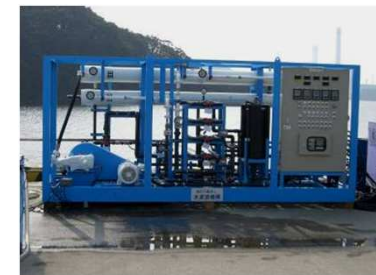
Mobile desalination unit
