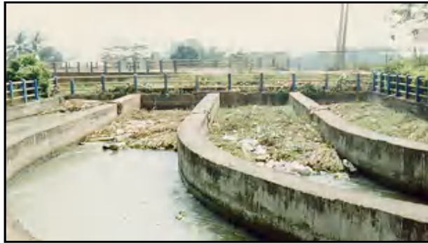
Debris in Cibeeet Syphon
