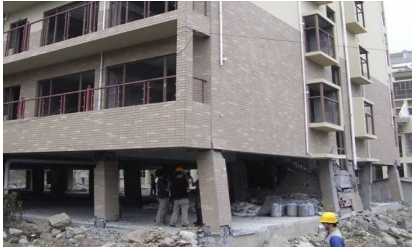
Partially damaged concrete building
