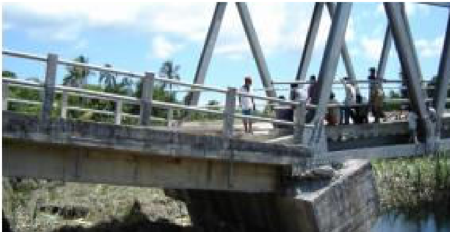
A bridge damaged by soil liquefaction (March 28, 2005)
