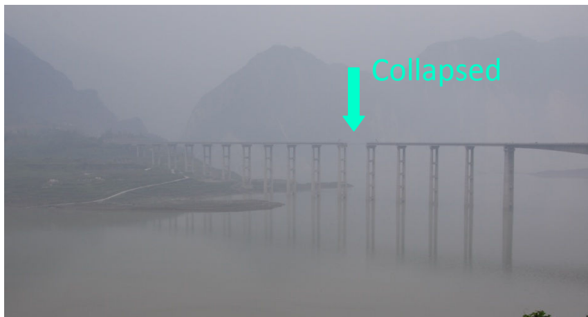
Fallen concrete girder of a bridge
