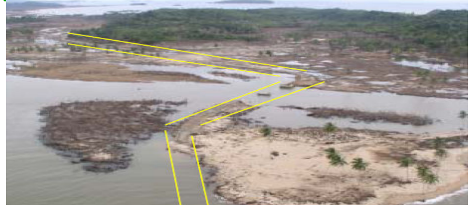
Roads along the coast were washed away and largely subsided
