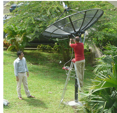
GNC Receiving Station
